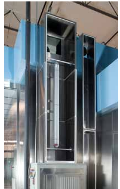
Figure 2: UVC Lamp Fixture Installed Inside Cleanroom Air Return (shown with cover removed)
