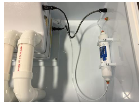
Photo 5. Drain Pan with ball valve
