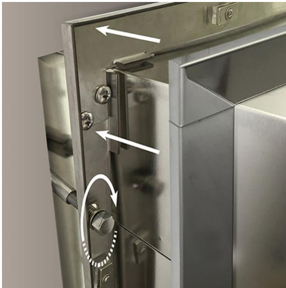
Figure 7: Thread the lag bolt into the guide attached to the “clean”-side bracket, sandwiching the wall between the brackets
