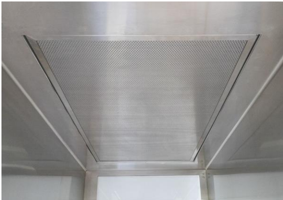
Figure 15: A stainless steel screen hides the HEPA filter
