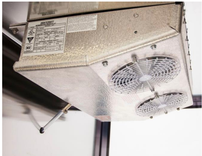
Figure 21: Drain tube exiting the evaporator inside the pass-through
