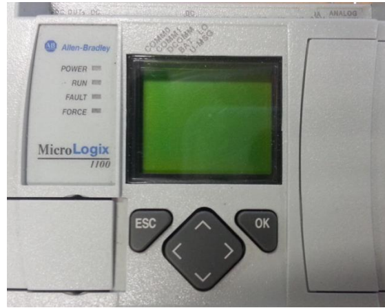
Figure 8: Internal PLC Panel
