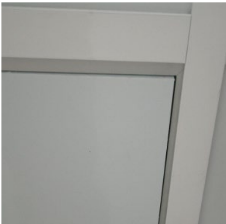
Figure 13: Panel fully attached to filter screen without overlapping edges
