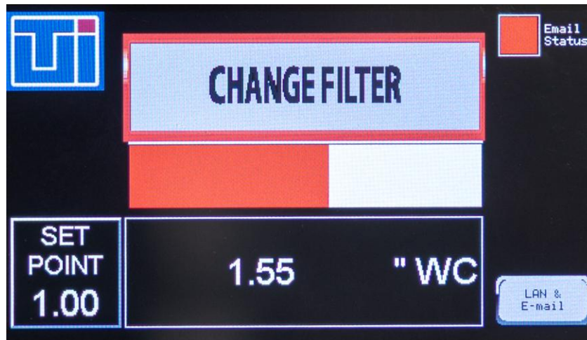
Figure 4: Alarm state — CHANGE FILTER triggered at 1.55" WC
