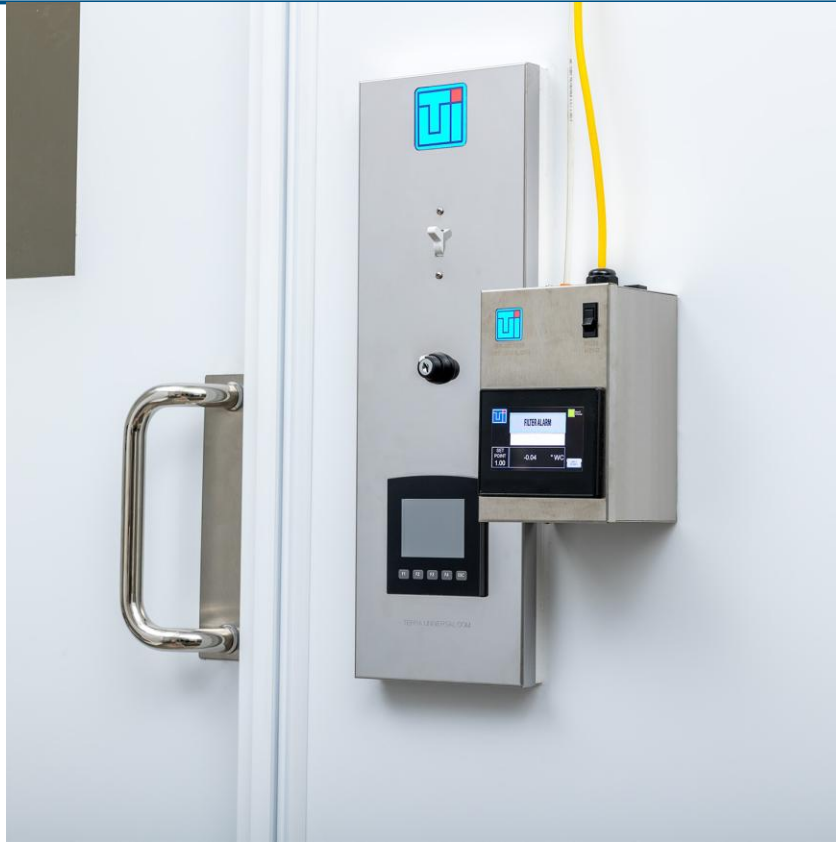
Figure 2: Unit installed at cleanroom entry
