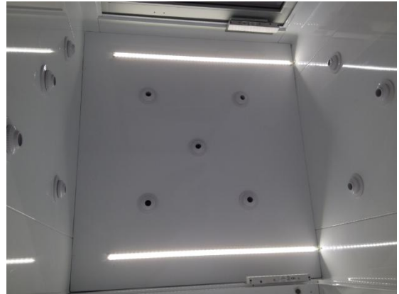
Photo 32: Typical Air Shower/Tunnel LED lighting
