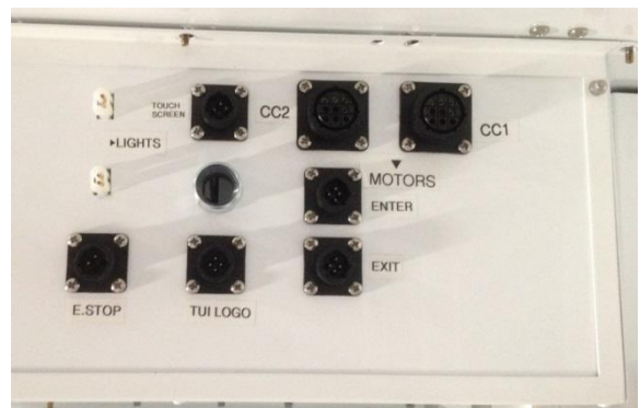
Photo 17: Main Junction Box Connections Panel
