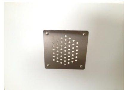
Photo 6: Make-up air vent
