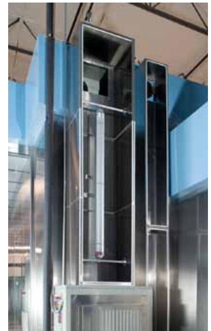
Figure 2: UVC Lamp Fixture Installed Inside Cleanroom Air Return (shown with cover removed)
