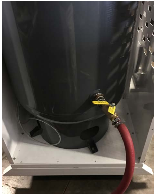
Figure 3. Inlet Valve on Compressed Air Storage Tank (shown with side panel removed)
