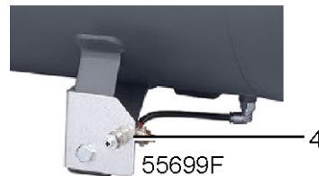
Figure 70: Condensate drain valve on air receiver
