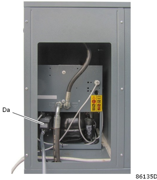
Figure 47: Automatic condensate drain
