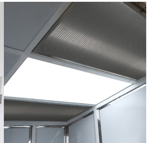
Cleanroom LED lights are energy efficient, produce low heat, carry long life spans and are compatible with ISO class 3 spaces
