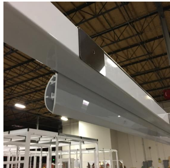
Figure 5: Grip Track bracket hooked onto the frame (view from inside the cleanroom)
